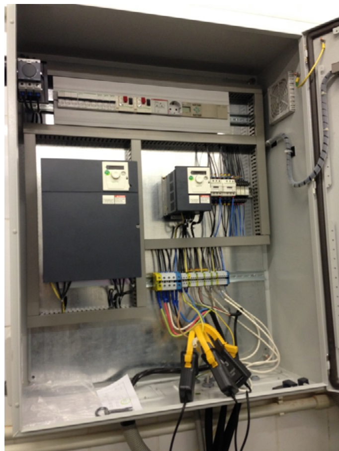
Figure 1 - IBF-1 control cabinet
